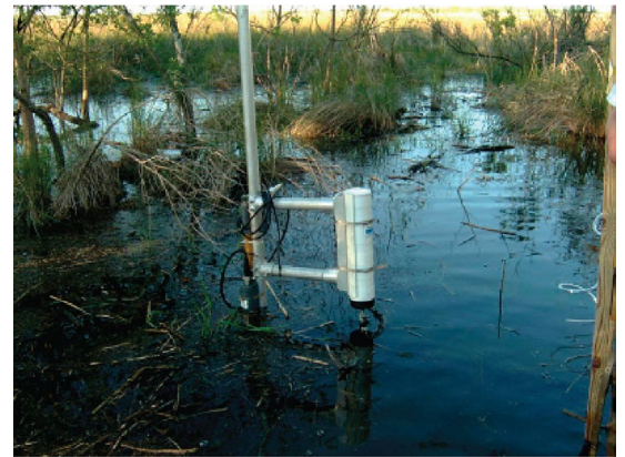
This LSU station utilized an Argonaut-ADV and a YSI sonde to gather data on flow and water quality. The data are invaluable tools as hydrologists and policymakers discuss how to better manage Louisiana's shrinking wetlands.
